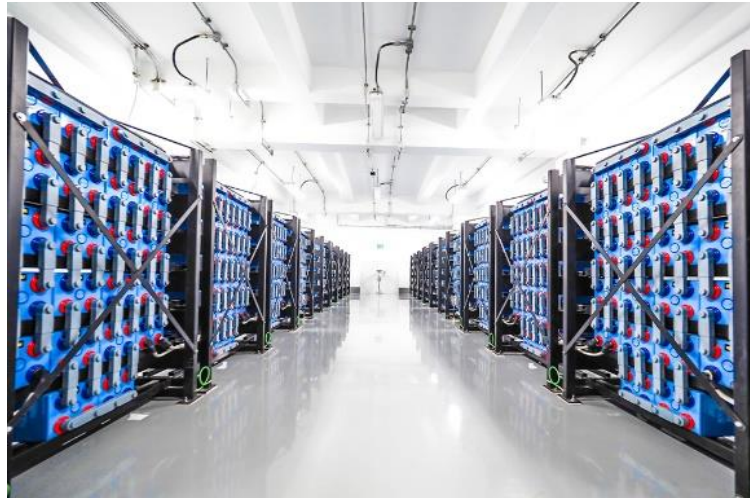
Figure 7 An example of an energy storage system using a battery
