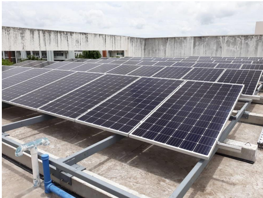
Figure 1 The roof-top area of the Administration Building, Faculty of Science, Naresuan University
