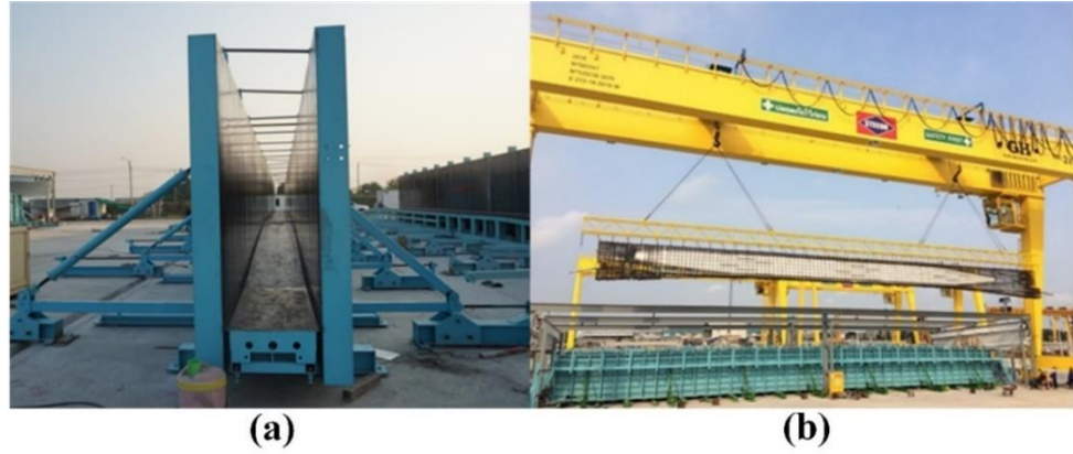
Figure 85 Construction details of the monorail girders: (a) formwork and (b) installation of the steel cage.
