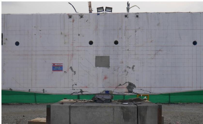
Figure 164 Cracking pattern at the pier segment.
