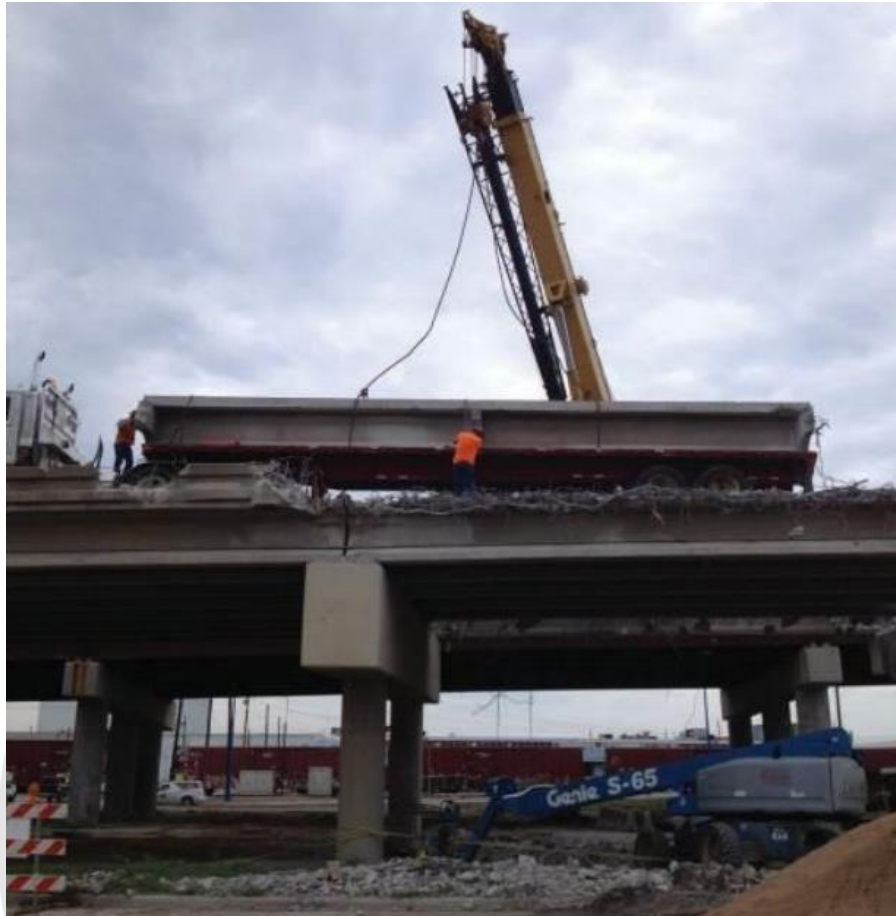
Figure 29 Removal of girder C from the I-244 bridge over the Arkansas river in Tulsa, OK on September 4, 2013 (photo courtesy of Gary Quinonez with Manhattan Road & Bridge) [34]
