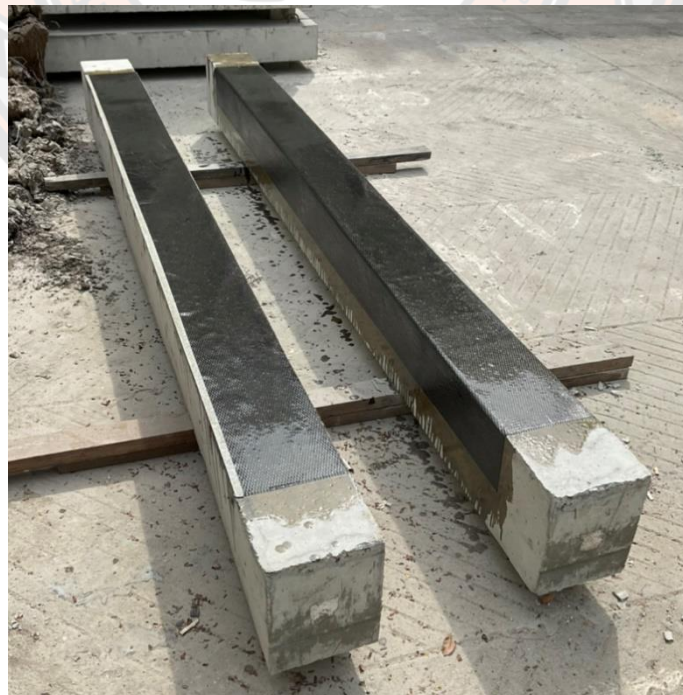
Figure 105 Application of CFRP sheet on bottom of beams (left) tension side only (right) u-shape sheet
