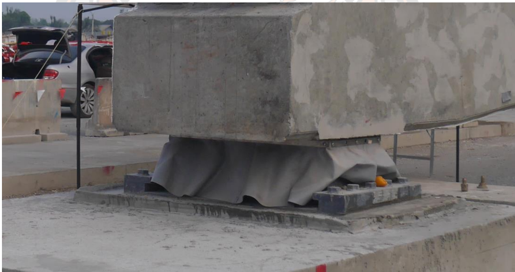
Figure 159 Bearing B-04 after test
