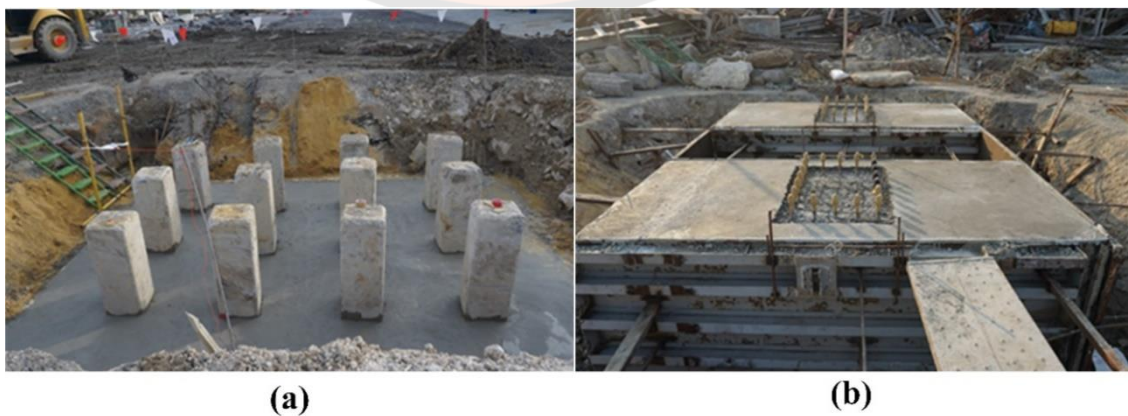
Figure 87 Construction details of the foundations (a) pre-cast piles foundation, and (b) pile caps.
