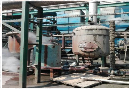
Blow down tank
