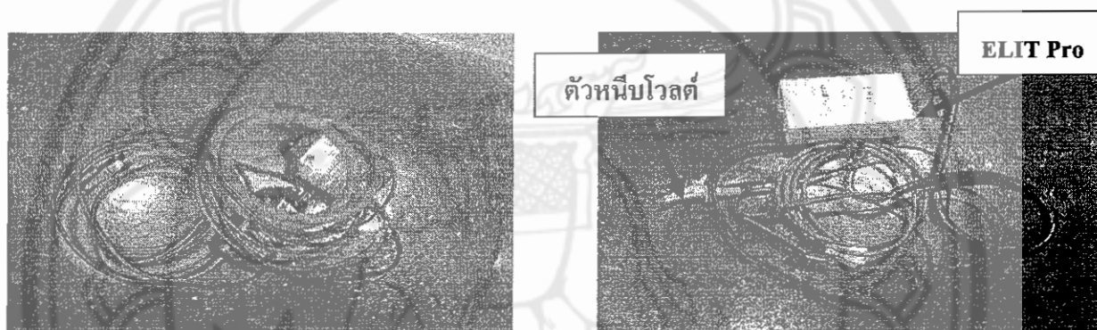
ก.แสดง CT (Current Transformer)
